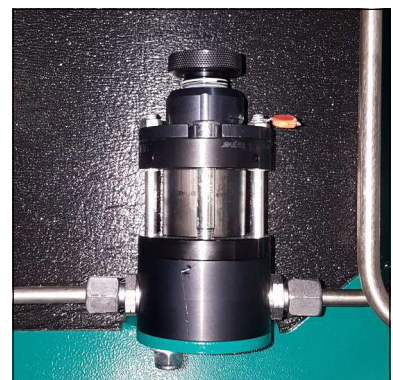
Safety valve 4th stage
