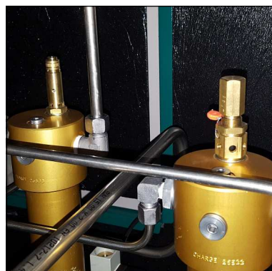
Safety valve 2nd and 3rd stage
