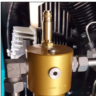
Safety valve 1st stage
