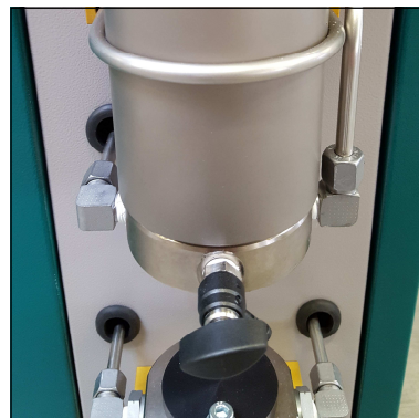
Fig. 3 - Loose pipe connections and nuts
